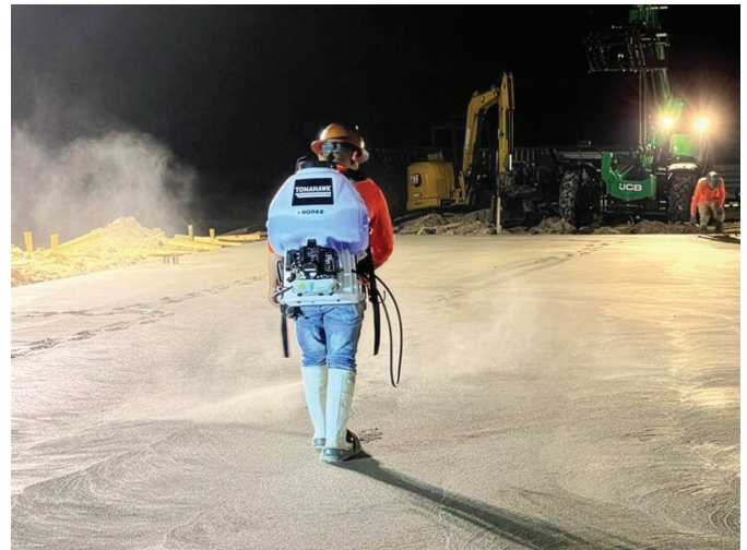
Fig. 2: Based on real-time measurements, concrete contractors should adjust their setting procedures. Here, a worker entraps bleed water on the concrete surface under a uniform film of a liquid applied evaporation retardant. It is critical to apply the evaporation retardant after strikeoff and between the different floating operations (photo courtesy of Ben Wiese)
